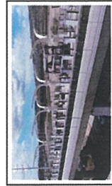
Crews continue to make progress in completing the nine stations across the Ewa-end of the Honolulu Rail Transit Project.
