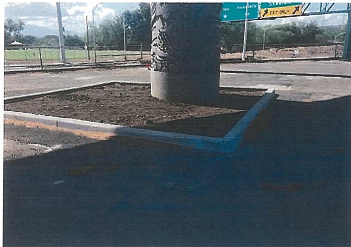
Curb area at HART Pier requiring topsoil
