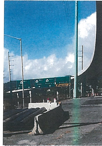
New HECO Power Pole in Bus Lot
