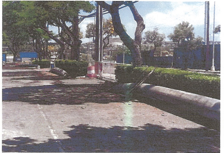
Force main Bypass in bus lot
