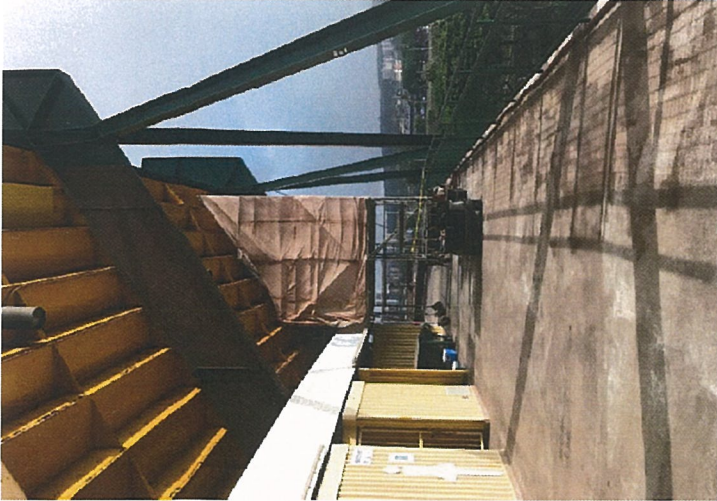
Movable Scaffold used to removal loose rust and Fibreglas angles (Yellow LL-QQ)
